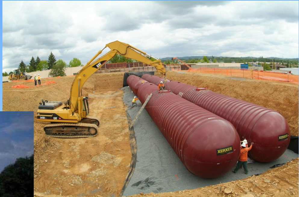
Underground fiberglass tanks
